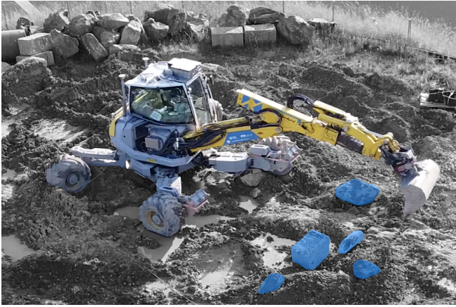
Fig. 1: Example excavation scene with rocks of varying shapes, sizes, and surface conditions (target rocks highlighted in blue). Reliable detection and removal of such objects is critical for safe and efficient downstream tasks like terrain leveling or continued excavation.
