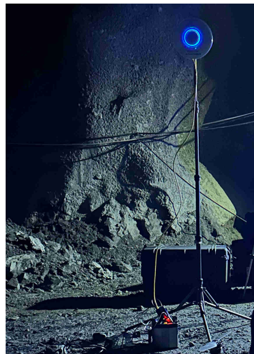
Fig. 13: One of the nodes in the mobile Wi-Fi mesh used to provide communication for the task coordination. The Ubiquiti U6 Pro is mounted on a tripod and connected to a battery to allow for easy and quick deployment in the underground environment.
