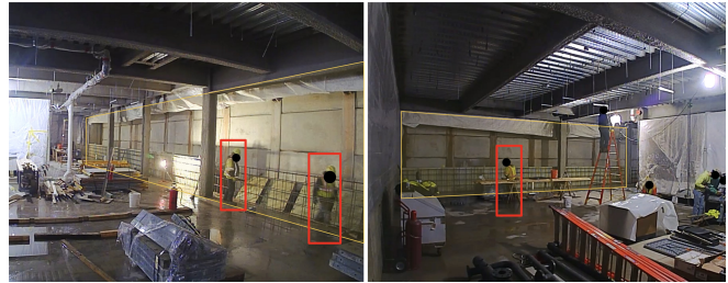
Fig. 1: Site observation captures of the carpentry formwork activity and construction site condition
