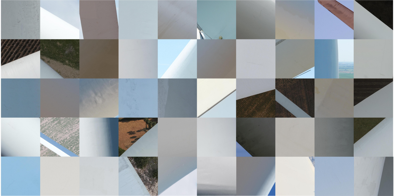
Fig. 1: Can you spot the cracks in these images? Hairline cracks are barely visible and commonly confused with stains and markings from dirt or grease. However, these defects can lead to catastrophic and irreparable damage to wind turbines if left untreated. This figure contains sample tiles from our Zeitview Crack Detection (ZVCD) dataset of annotated barely-visible surface cracks collected from inspections across the globe. This dataset is used to train our turbine crack detection pipeline for the inspection of renewable wind energy sources.
