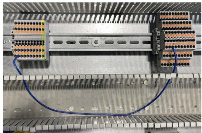
Figure 1. Picture of a typical wiring task, where two terminal blocks are connected by a wire. The middle piece of the wire is routed through a wire duct.
