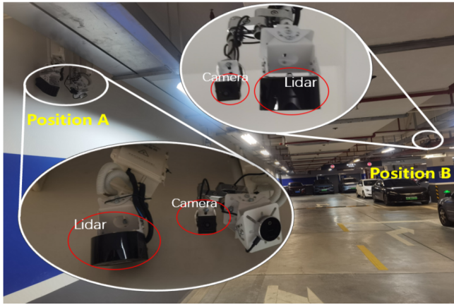
Fig. 4. Scene Installation Diagram. Two sets of infrastructure LiDAR-camera pairs are installed at positions A and B, respectively, and positions A and B are located on both sides of the parking lot road and towards the parking lot ground.
