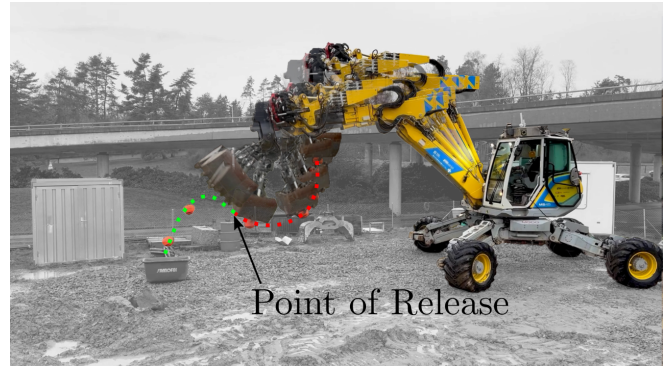
Fig. 1. Two-dimensional throwing controller deployed on the M545 excavator with overlaid payload trajectory.
