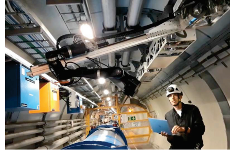
Fig. 2. The Train Inspection Monorail (TIM) in the LHC tunnel.
